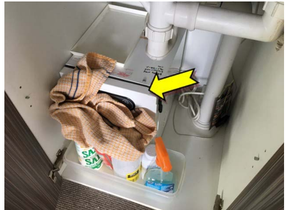
Photo 4. Interior, upper level, meeting room, under sink, hot water heater – suspected SMF-containing internal insulation material.
