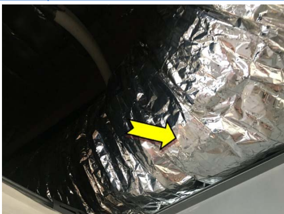
Photo 5. Interior, upper level, eastern end of meeting room, ceiling space, ductwork – suspected SMF-containing internal insulation material.
