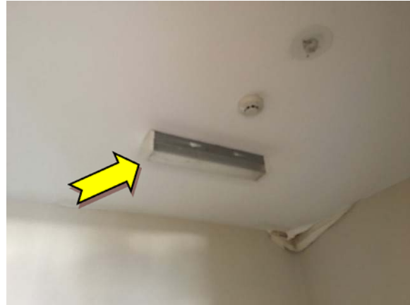
Photo 8. Interior, ground level, storage cupboard, single tube fluorescent light fitting – suspected PCB-containing capacitor.
