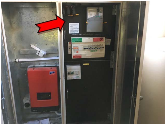
Photo 3. Interior, ground level, main hall, electrical cupboard, electric backing board – suspected asbestos-containing bituminous backing board.
