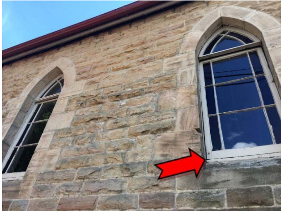
Photo 1. Exterior, ground level, throughout, window frames – suspected asbestos-containing window caulking.
