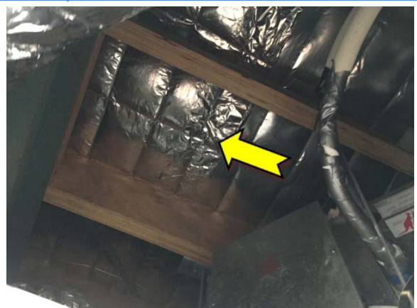
Photo 6. Interior, upper level, eastern end of meeting room, ceiling space – suspected SMF-containing sarking insulation material.
