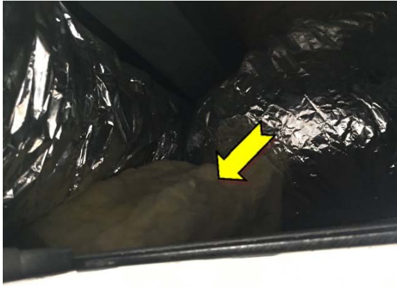
Photo 7. Interior, upper level, eastern end of meeting room, ceiling space – suspected SMF-containing insulation batts material.
