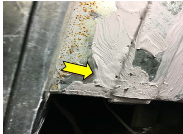
Photo 2. Interior, ground level, toilet, ceiling space, duct – suspected non asbestos-containing mastic sealant.
