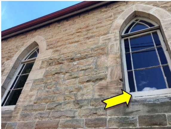
Photo 9. Exterior, throughout, window frames – suspected lead-containing cream upper coloured paint system.
